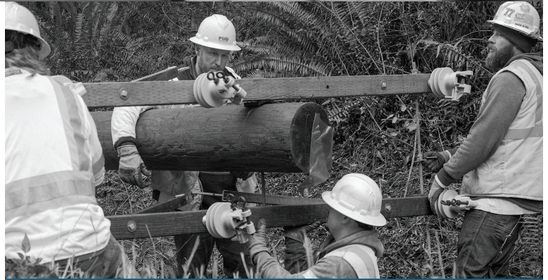
Line crew install a dual crossarm assembly to a new utility pole.
