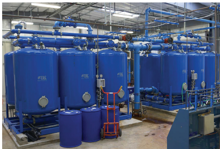
Sparling well treatment plant near Hadlock
